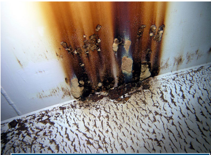
Rust tubercles along the floor to wall weld seam exhibiting the rust staining.
