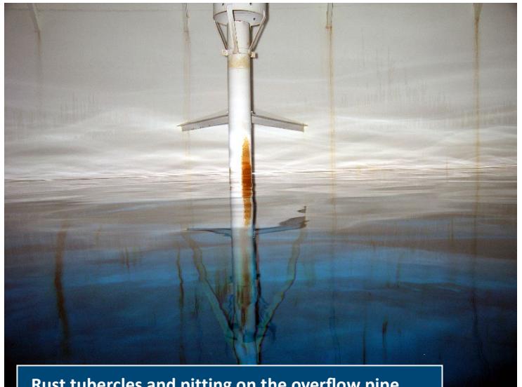
Rust tubercles and pitting on the overflow pipe.
