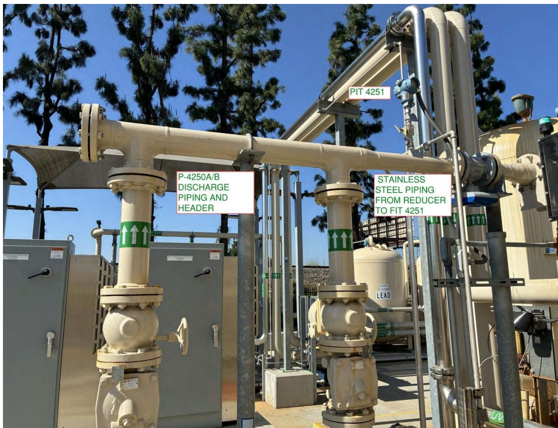
Figure 1: P-4250A/B Discharge and Stainless Steel from Reducer to FIT-4251 (CPVC Replacement Prior to Reducer and Stainless Steel After Reducer)
