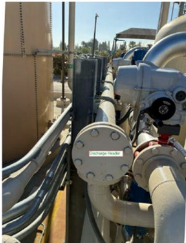
Figure 5: Header & Process Pipe to MMF System, Blind Flange (CPVC Replacement)
