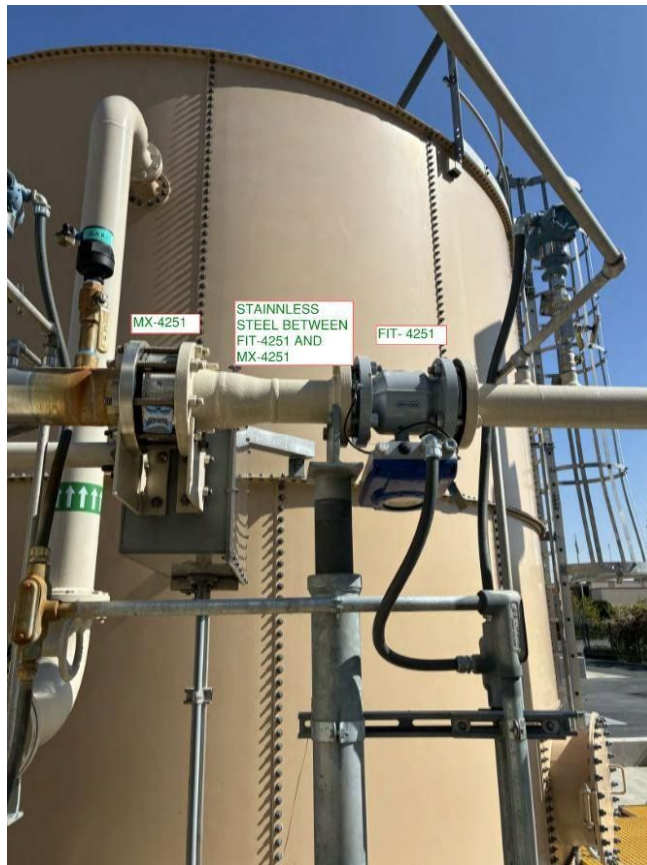
Figure 4: Stainless Steel Piping from FIT-4251 to MX-4251 (Alternate View)
