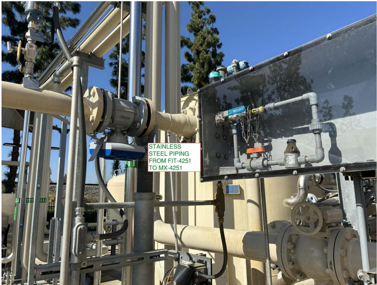
Figure 2: Provide and Install SS 304L Schedule 40 Pipe Spool Piece from FIT-4251 to MX-4251
