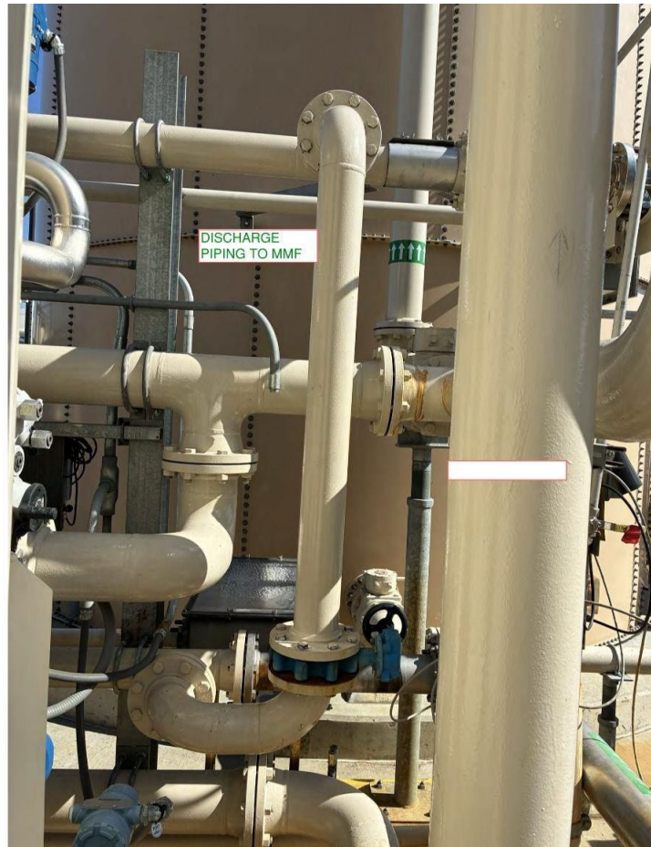
Figure 3: Discharge Piping to MMF (CPVC Replacement)
