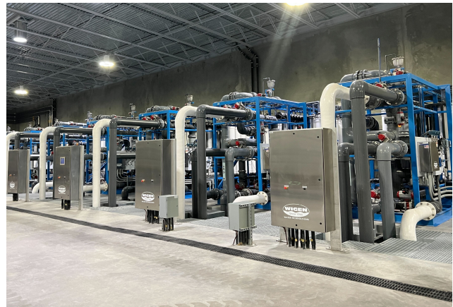
UF Trains at Pure Water Oceanside AWPF
